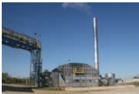
A new regenerative thermal oxidizer (RTO) installation at On-Cor's Wisconsin facility
